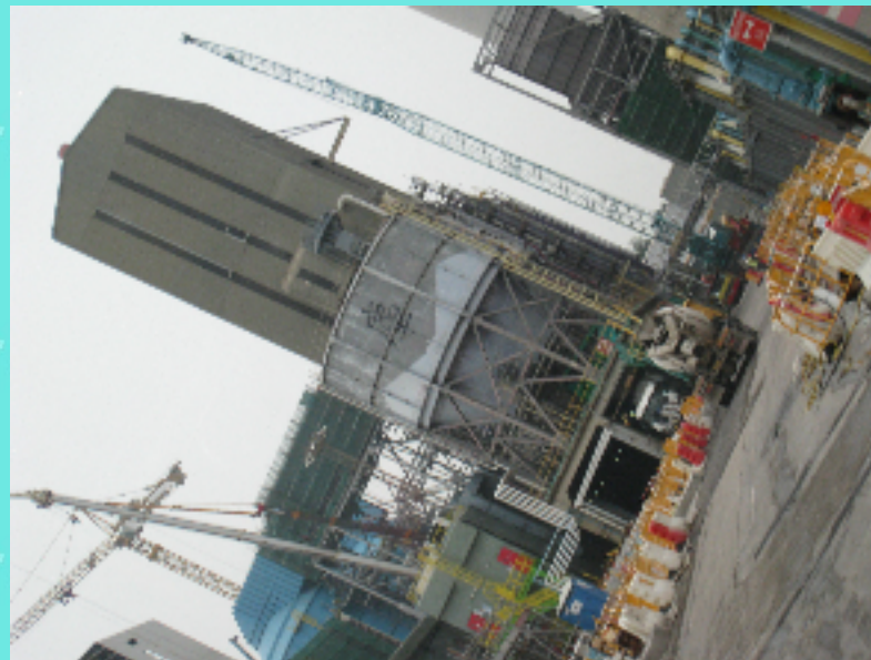
The dirt filtered out from the incoming air
