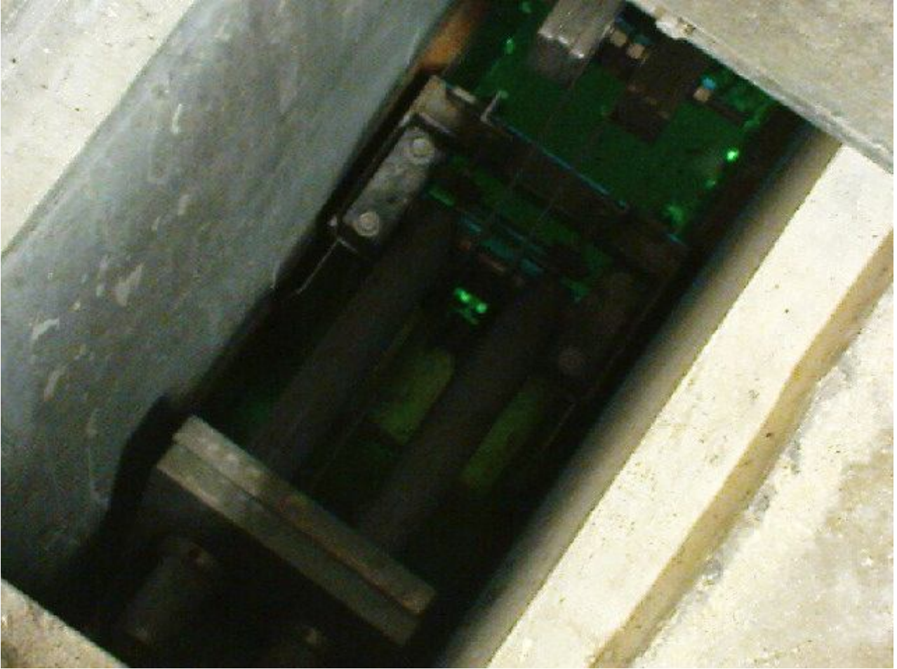
This photo shows a device in the UV disinfection process. UV disinfection is a part of tertiary sewage treatment, which is first used in Ngong Ping Sewage Treatment Works.
