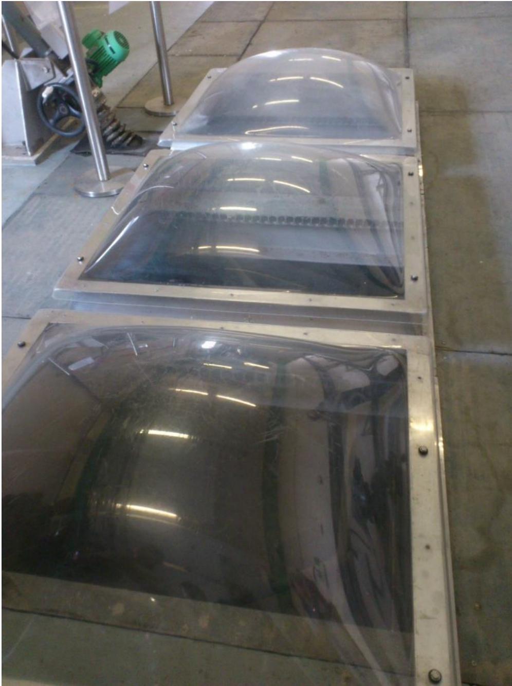
This is a Sequencing Batch Reactor technology (SBR). It is a Secondary Treatment used to remove organic matters and part of the nutrients.
