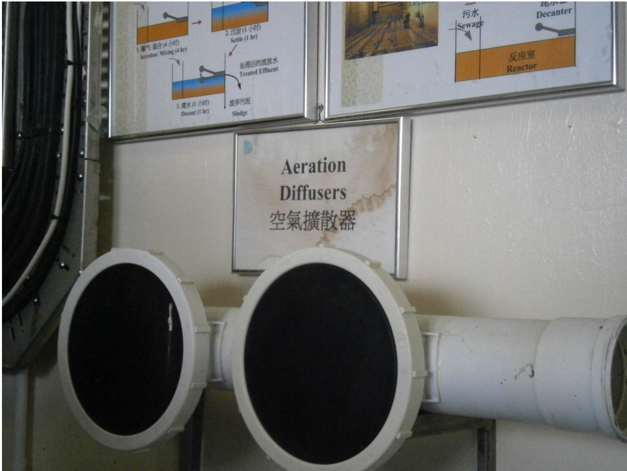
This is the aeration diffusers. It is used to produce air bubbles for trapping the oil in the water during the sewage treatment.
